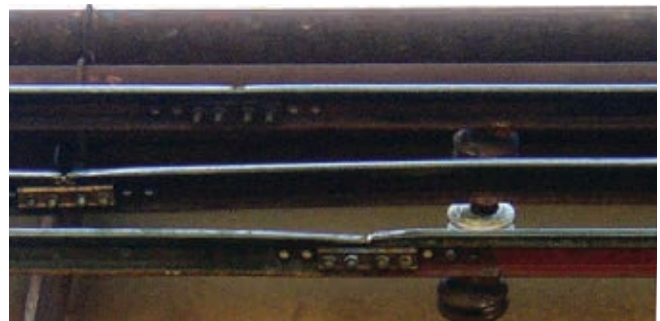
An example of excessive wear due to electrical erosion at the steel conductor bar joints.
